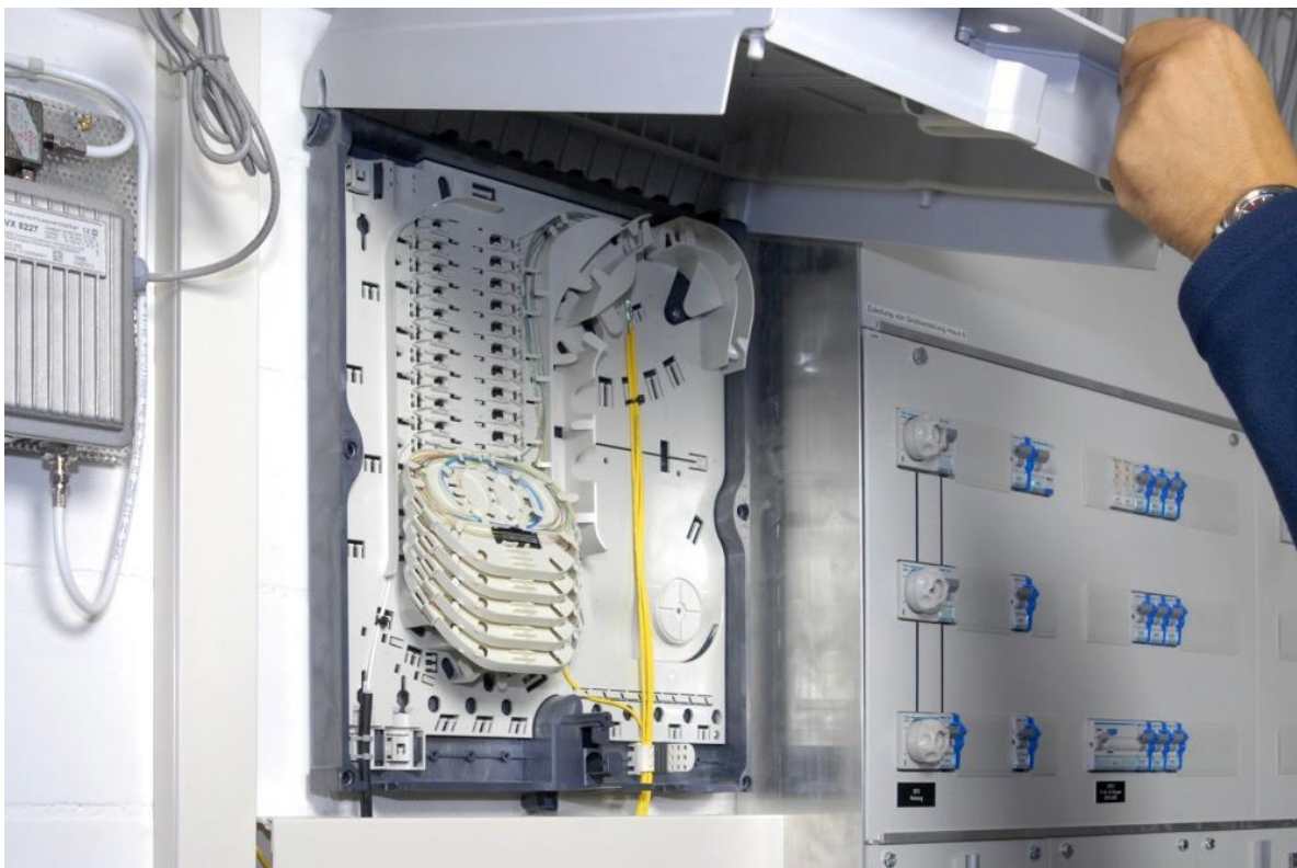
Figure 50: Example of wall mounted BEP installed next to a power distribution
