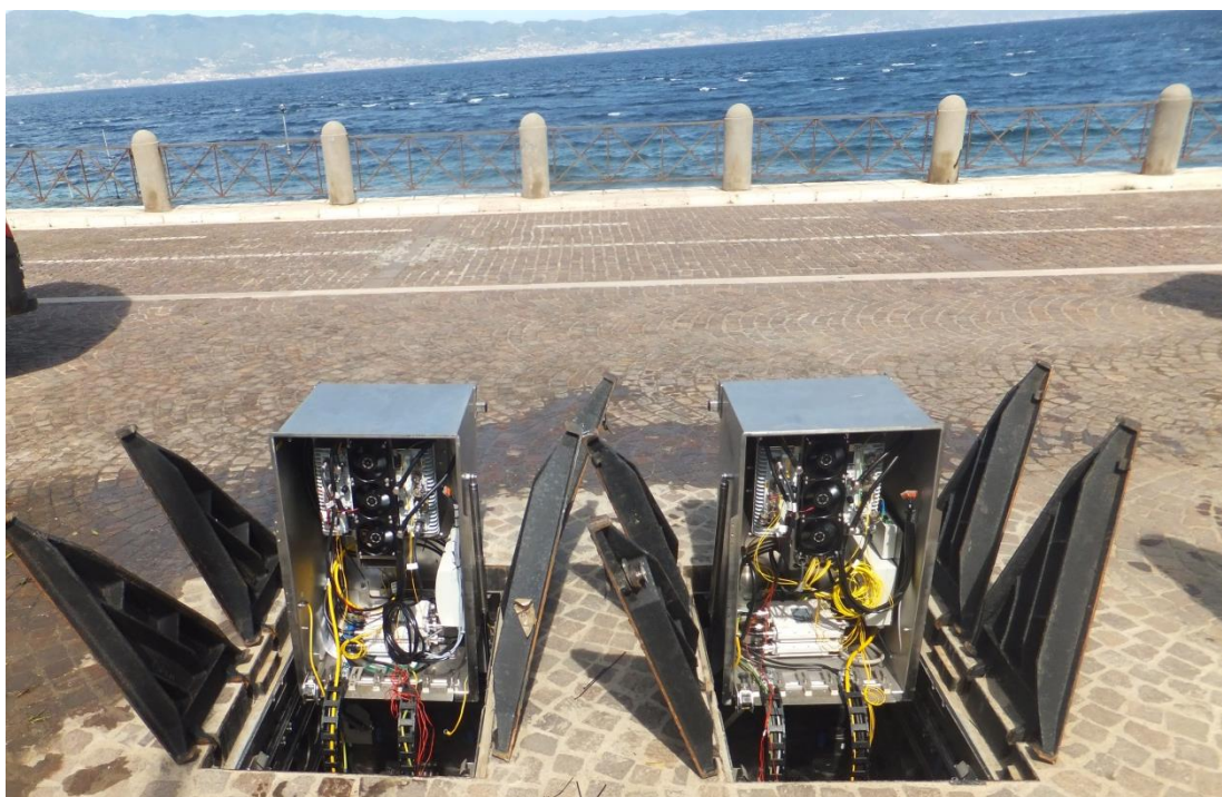
Figure 130: Underground Distribution System
