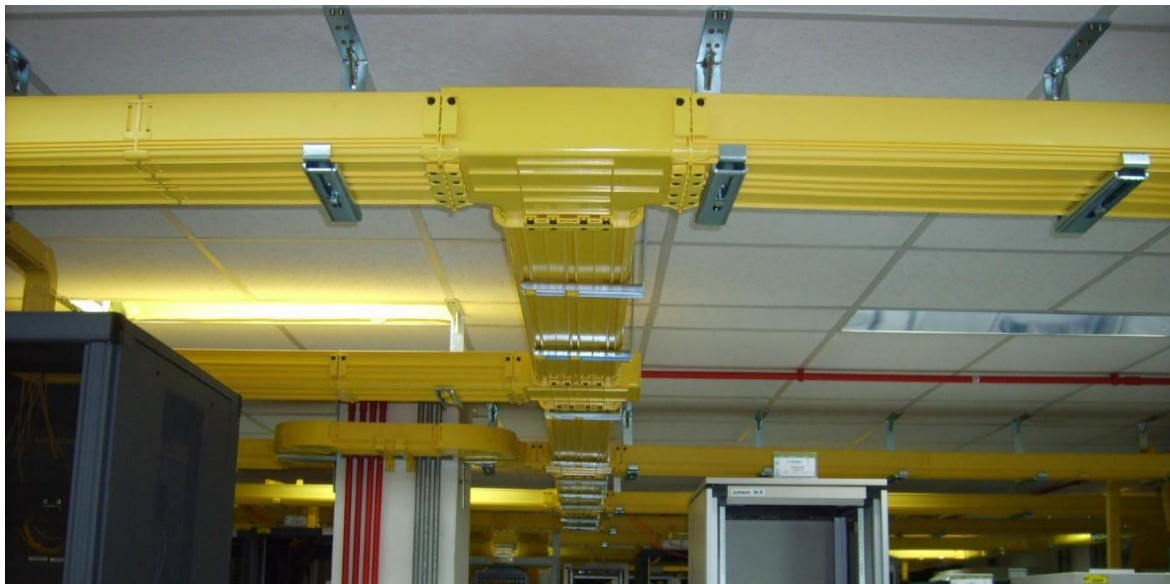
Figure 124: Examples of overhead fibre containment
