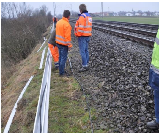
Figure 96a: Buckled cable after pushing too hard during blowing
