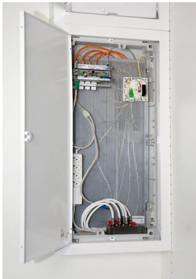
Figure 54: OTO integrated in a home distribution cabinet
