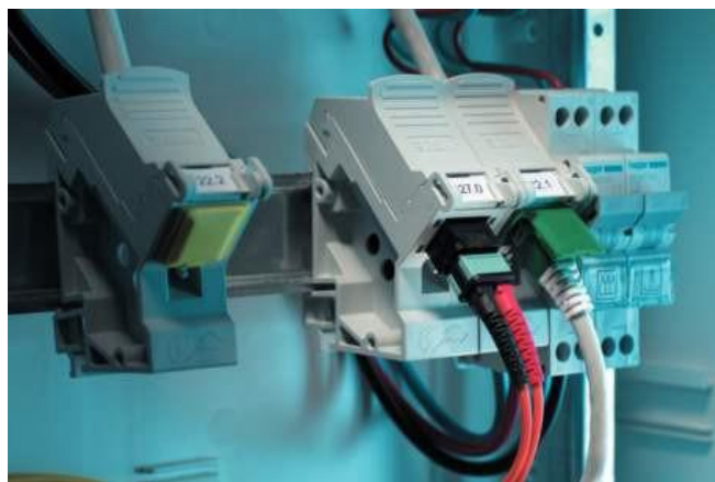
Figure 55: OTO integrated in the home electrical distribution panel
