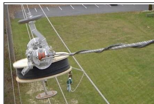
Figure 105: Wrapped aerial cable
