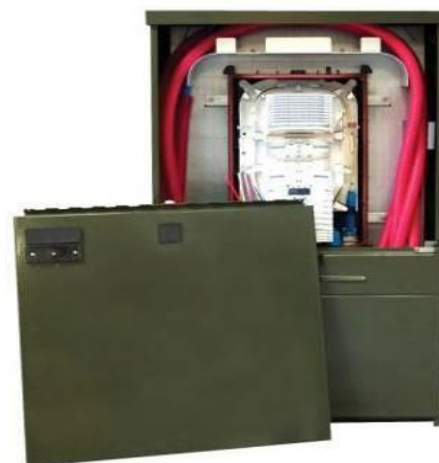
Figure 127: Typical street cabinet
