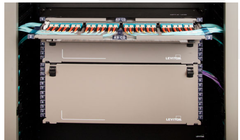
Fiber patching, 144 fibers per RU
